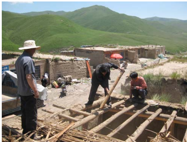
One of the trainees dismantles the old adobe structure. In its place, we built a brick and cement building to house the motorcycle repair shop.
